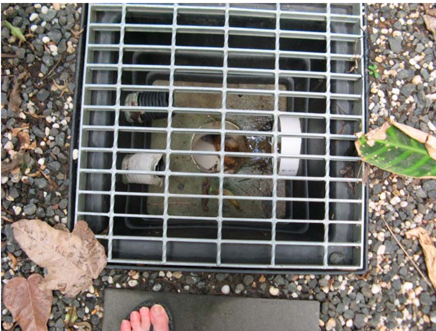
One of smaller grates giving access to the stormwater drain around Aura
