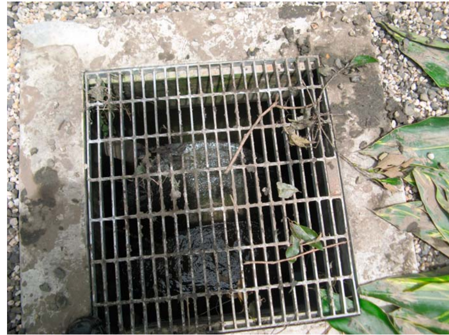
The large grate giving access to the stormwater drain at the side near the footpath gate on 14/01/11 at 1.04 pm, which can drown a person, if they fell in and could not get out
