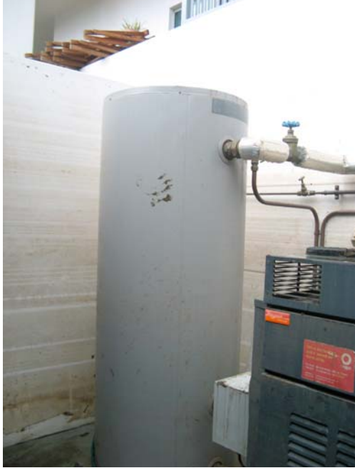
Water heaters that were completely submerged and damaged beyond repair
