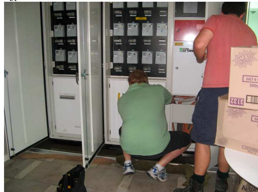
The main isolator switch on the power board was located at the lowest point on the panel and was the most expensive power component to replace
