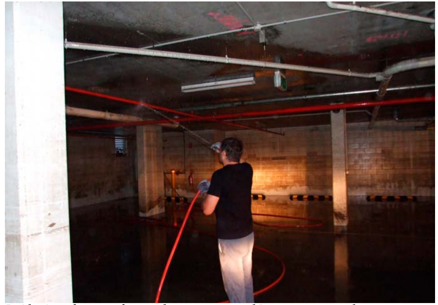
Inside view of one set of vents where water entered Basement 1 carpark
