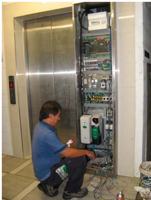
Aura lift control panel beside the lift in Basement 2 positioned at the lowest point in the building
