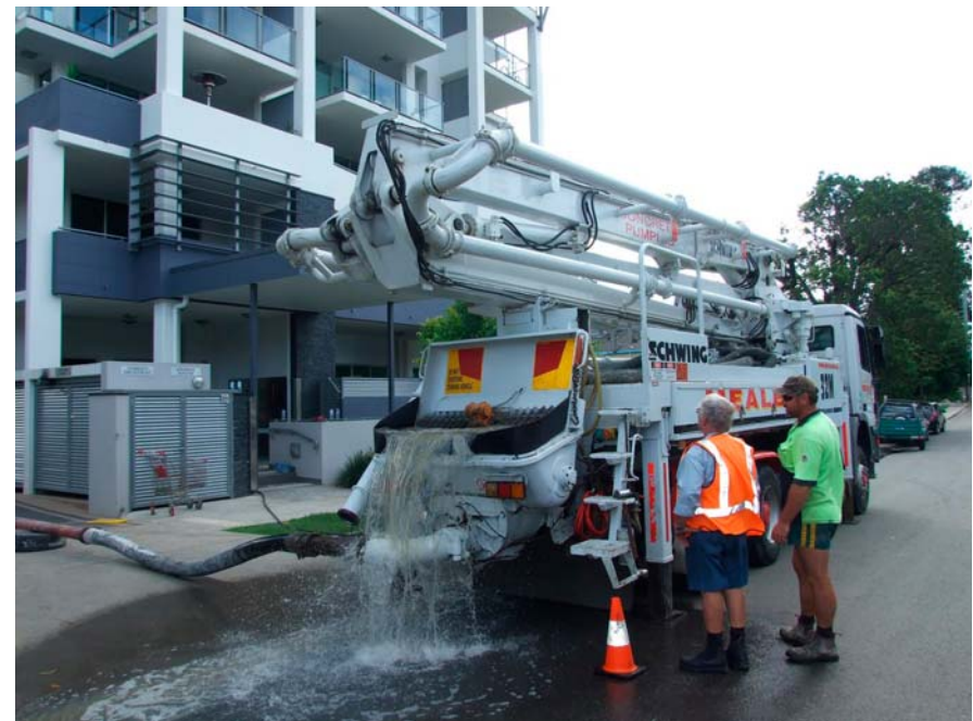
Pump truck needed to pump out Basement 2
