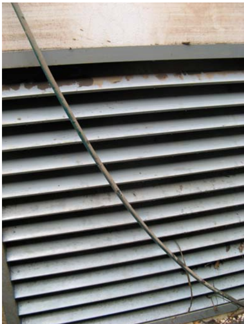
Close up of vents where water spilled into the B1 carpark basement
