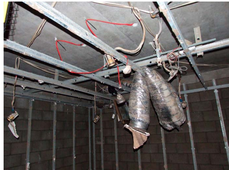
Part of the CO 2 monitoring system
