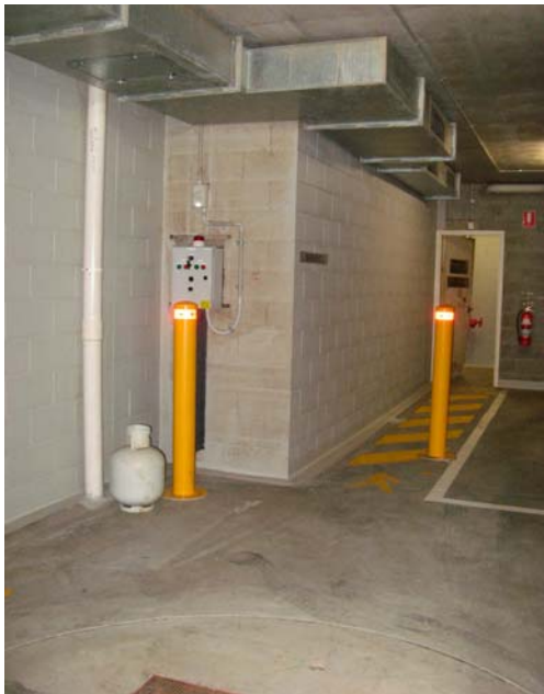
De-watering pump controls in Basement 2
