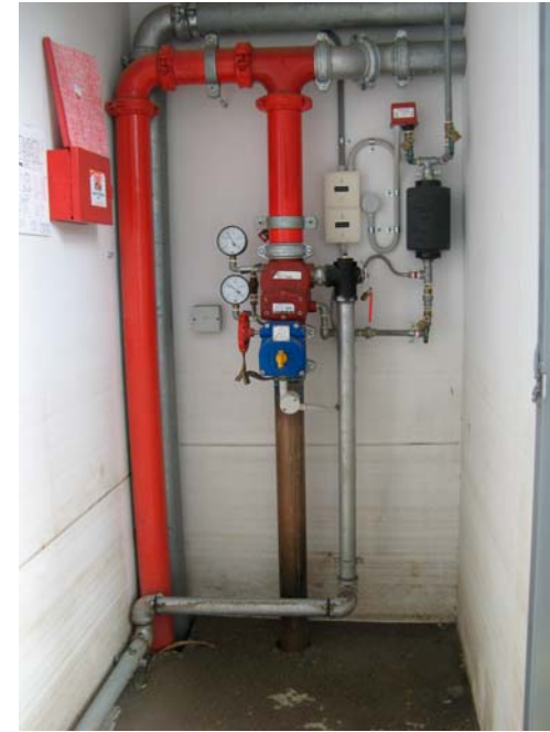
Inside the fire sprinkler system that was damaged by water
