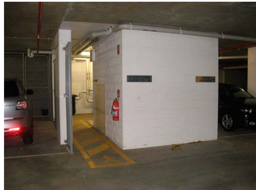
Lift well in Aura in Basement 2 with the main lift motor behind the yellow door in the wall near the fire extinguisher
