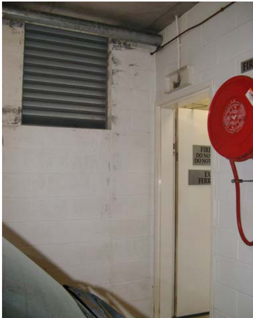
Basement 1 vents where water entered carpark
