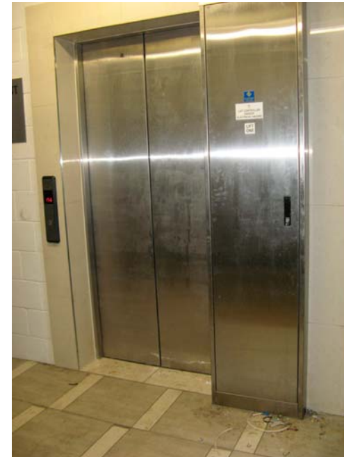
Aura lift doors on Basement 2 with controls on the right
