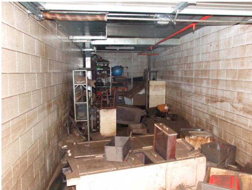
Metal ducts in the roof are part of the CO 2 control system
