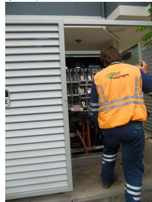
Energex inspecting transformer supplying electricity for Arriva and Aura
