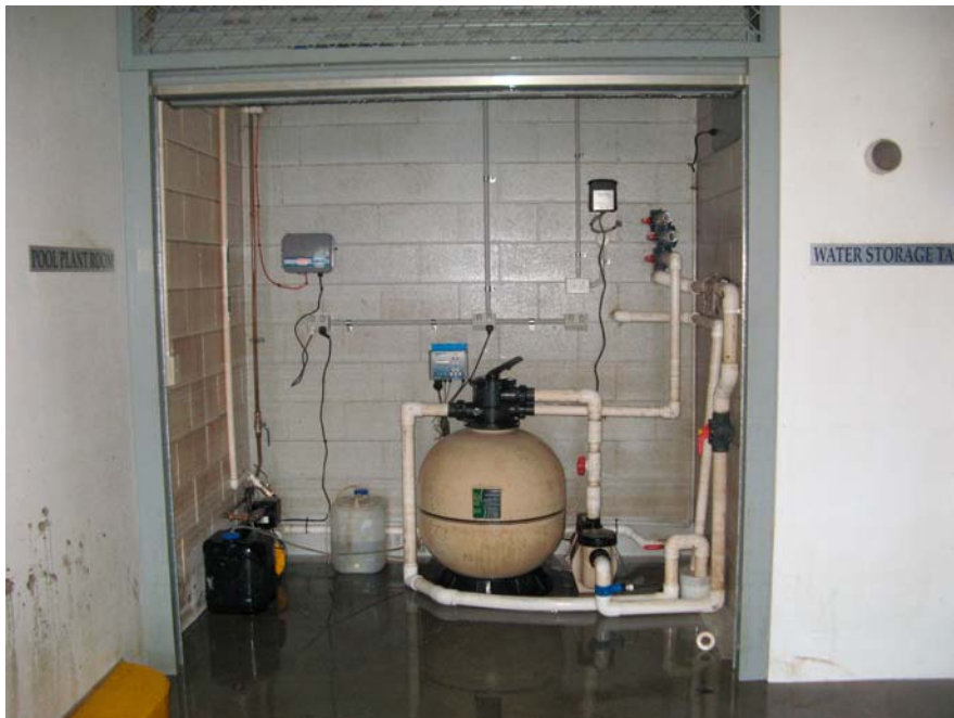
Close up of damaged pool controls in room with door raised on Basement 1
