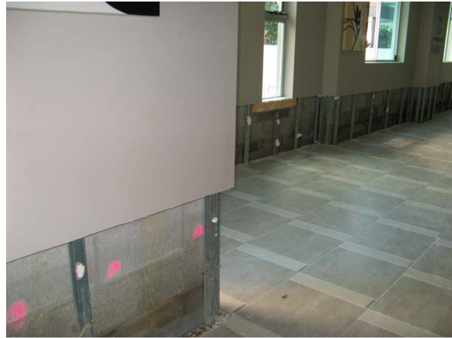
Damaged walls in the Aura foyer
