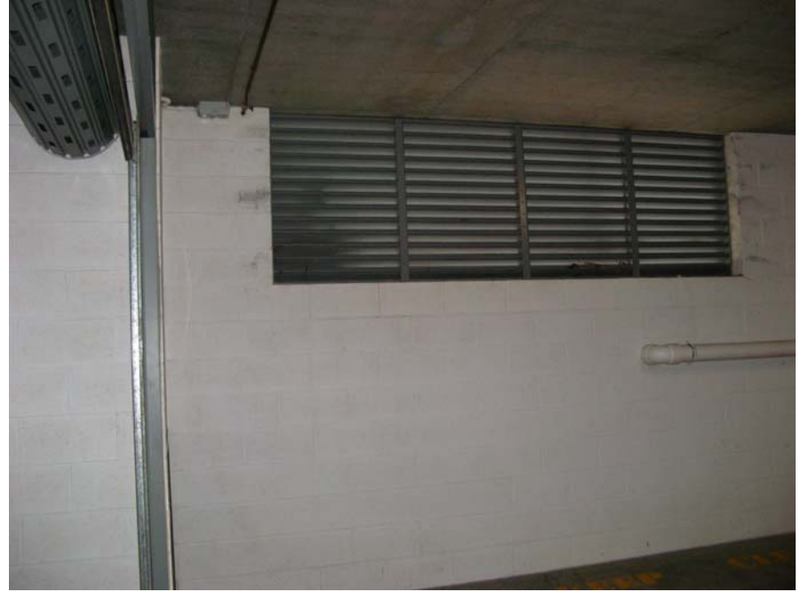
Basement 1 vents where water entered carpark
