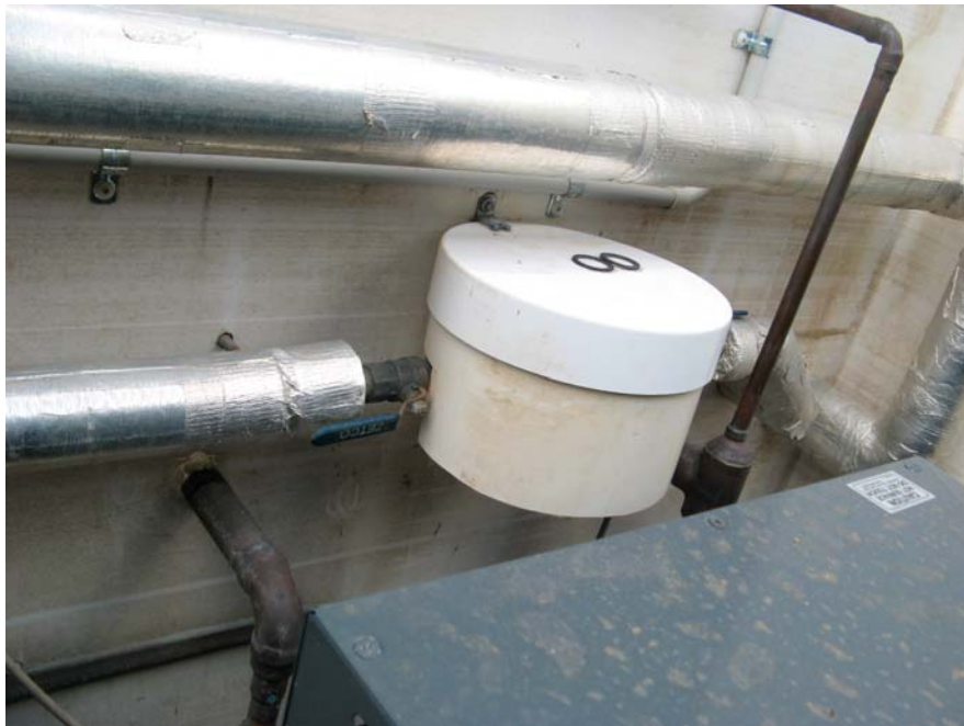
Hot water recirculation pump that cost Aura $450 to replace
