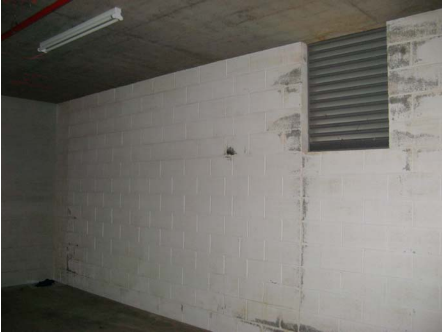
Basement 1 vents where water entered carpark
