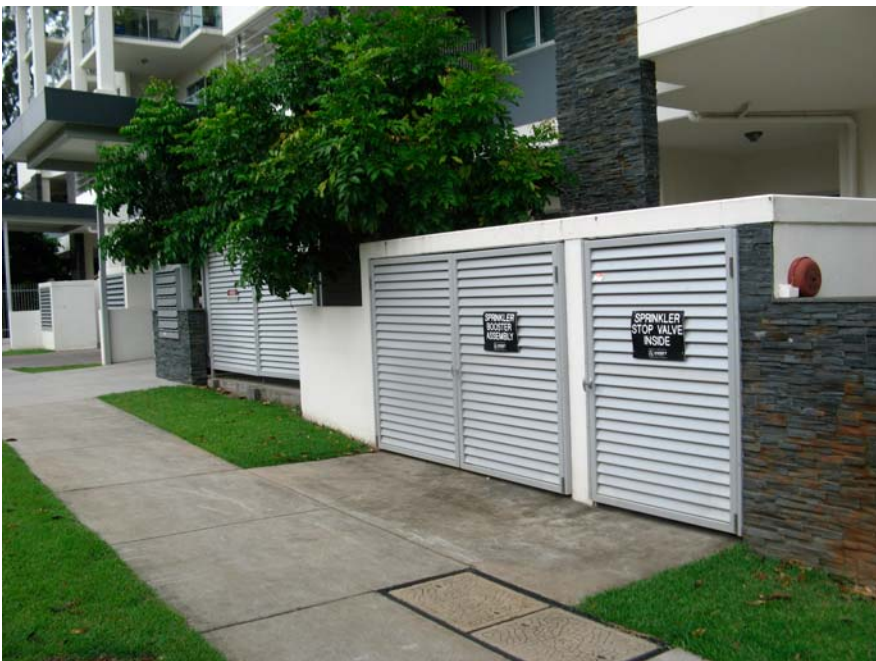
Room on left under tree housing Energex transformer for Arriva & Aura Apartments where water entered
