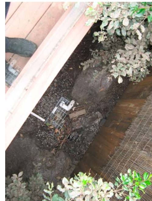
Aura stormwater drain on 14/01/11 at 2.53 pm showing where water bubbling up has not allowed any mud to settle around the grate
