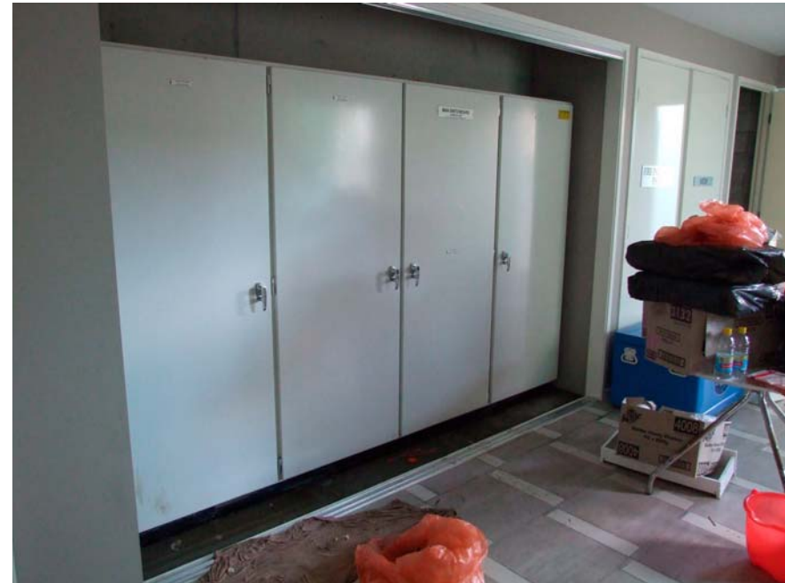
Power control panel inside Aura's foyer where partial damage occurred to the building power distribution.
