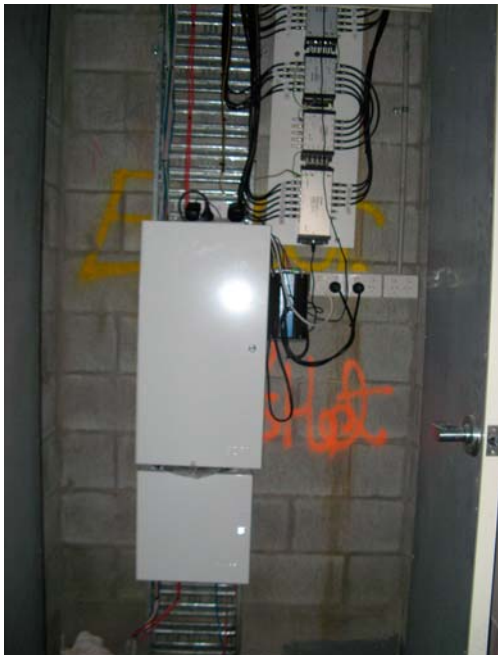
Video cabling controls located on ground floor
