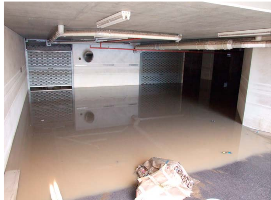
Aura carpark entrance showing room where pool controls are housed in room (left) on Basement 1
