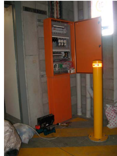
CO 2 Panel controls in Basement 1 beside the lift shaft
